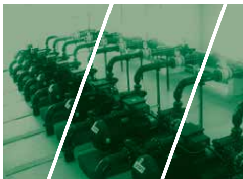
Boosting and Distribution of surface water
